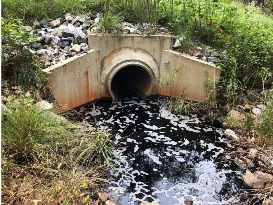
Photo 5. Stormwater retention pond outlet at the Franklin Generation Biomass Facility releasing black effluent into the Unnamed Tributary of Indian Creek. Photograph was taken by Anthony Rabern on October 6, 2019.
