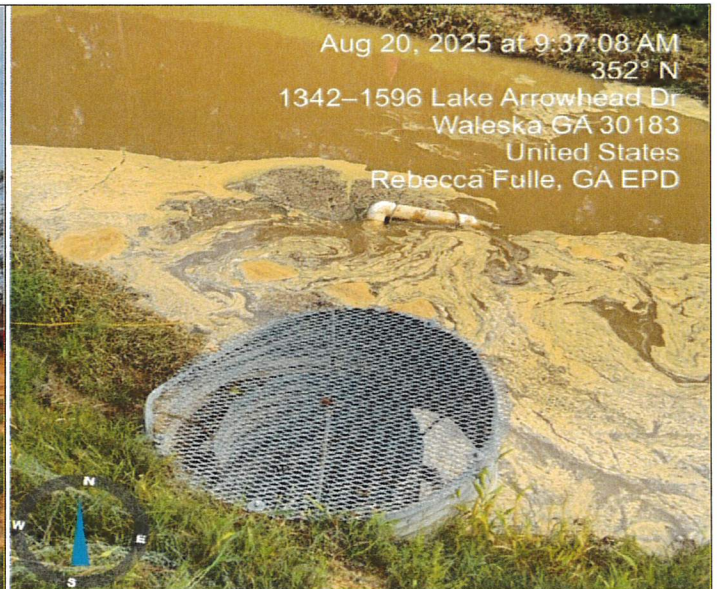
Photo Number: 4 of 6 Date: 08-20-25 Photographer: Rebecca Fulle Location: Site, facing North Observations: Surface skimmer requires maintenance.
