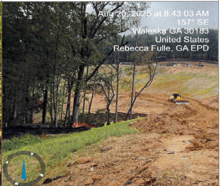
Photo Number: 6 of 8 Date: 08-20-25 Photographer: Rebecca Fulle Location: Site, facing southeast Observations: Land Disturbance Activity contributing to erosion and sedimentation issues.
