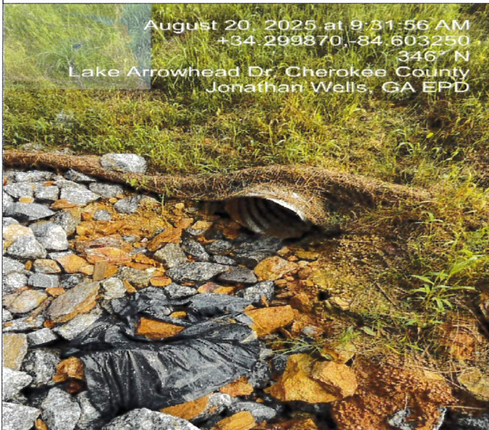
Photo Number: 5 of 8 Date: 08-20-25 Photographer: Jonathan Wells Location: Sediment basin outfall, facing North. Observations: Sediment observed leaving the site.
